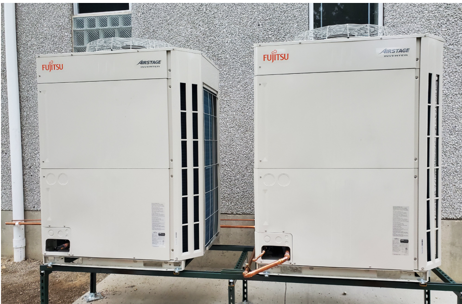
EcoWorks' new Fujitsu variable refrigerant flow (VRF) heat pump outdoor units. These units allow for each indoor unit to provide heating or cooling by adjusting the system's refrigerant flow.
