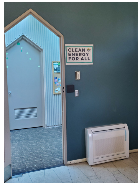
An indoor unit of the VRF heat pump system.
