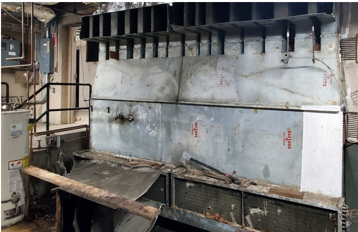
A view of EcoWorks' aging gas boiler prior to removal.
