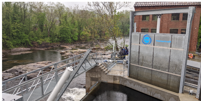
A look downriver over the dam's crest gate, which improves the turbine's efficiency and enhances recreational activities, such as kayaking, upriver.
